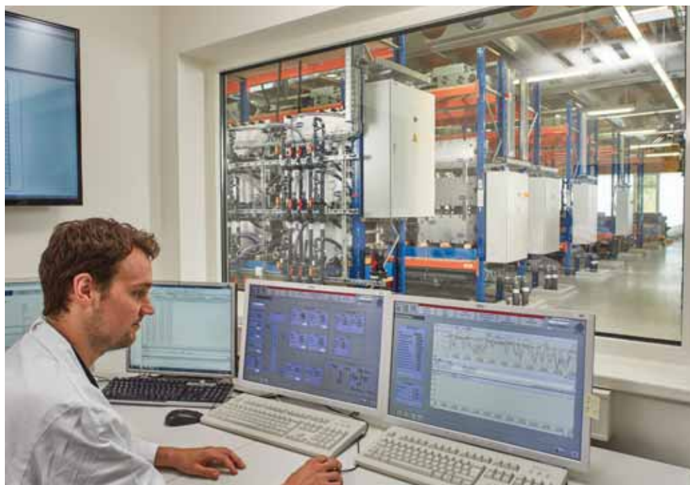
Figure 6. Control room of a 2 MW/20 MWh vanadium redox flow battery at Fraunhofer ICT
