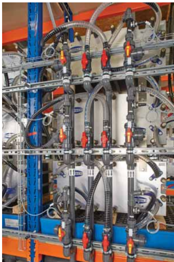
Figure 8. Piping and stacks of a 2 MW/20 MWh vanadium redox flow battery at Fraunhofer ICT
