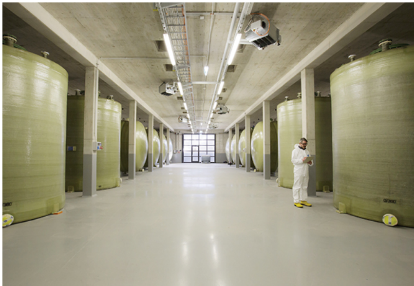
Figure 2. Shown here is the installation of the storage tanks that will hold acidic vanadium solutions for the 3-MW RedoxWind project in Pfinztal, Germany
